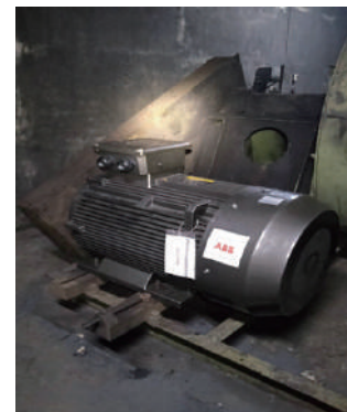
Jet cooling fans used at the APL cooling section Replaced high efficiency motors
